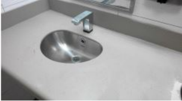
Description of Photo 3 : sensor operated sink faucet
